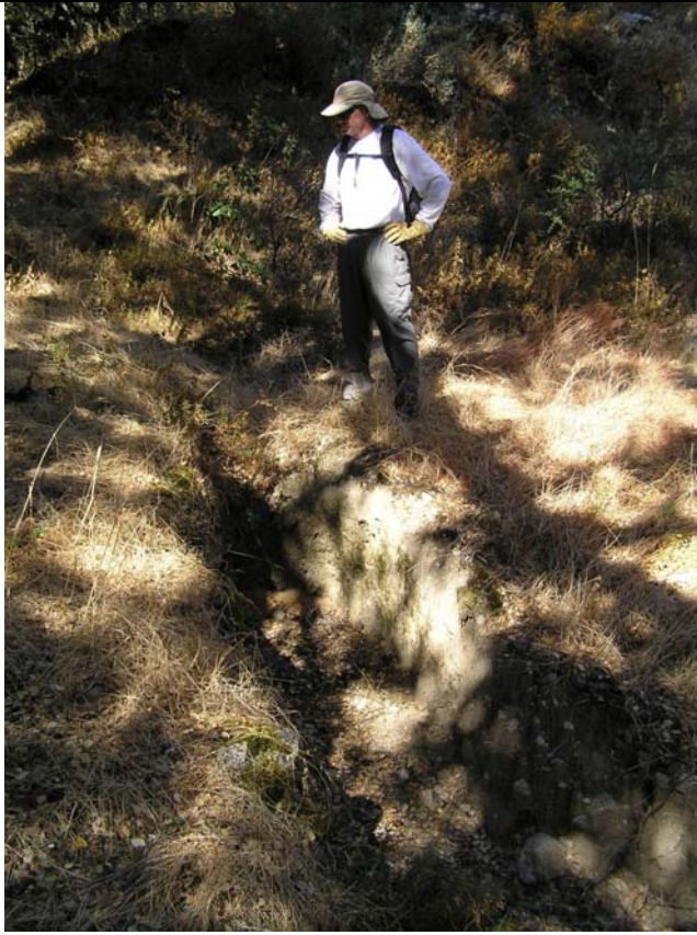
Headward erosion creating gully along Lopez-Perez Loop where road decommissioning may not have occurred in 1990/1991. Roadbed fill across small, ephemeral stream is being actively eroded and sediment is moving down-slope.
