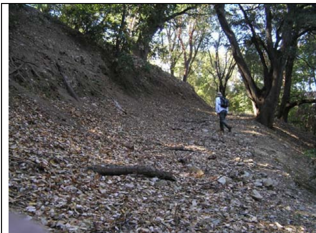
Decommissioned roadway is slightly out-sloped between upper section of Upper Wildcat road and Palo Corona Road. Out-sloping may be a function of natural soil and duff accumulation along inboard side of roadcut.
