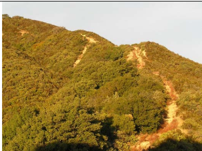
Extremely steep sections of Garrapata/Wildcat Ridge Road, with soil movement originating from improperly graded roadbed. Sediment is likely not being delivered to stream drainages, as this slide occurs upslope of densely vegetated Evergreen Forest and Mixed Chaparral habitat.
