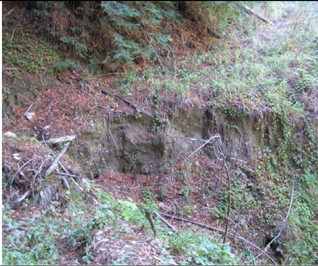
Location where fill of roadbed has failed leaving a 5-foot scour that may supply sediment during episodic events. Duff and redwood sorrel cover helps to mitigate potential future erosion at this location, however fill is unstable and may continue to erode.
