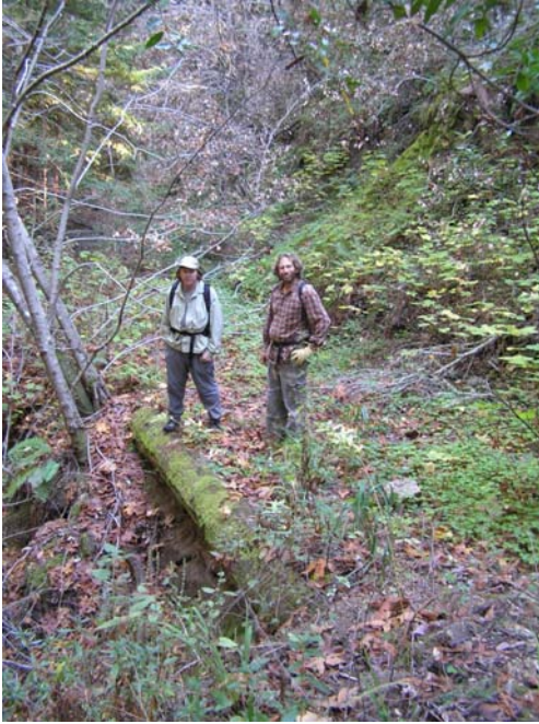
Very old bridge constructed out of redwood logs. No visible erosion is apparent along this reach of the road down into Wildcat Canyon. Redwood Forest supports a dense understory.
