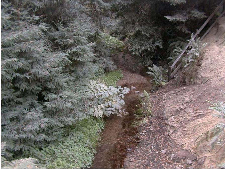
Figure 22 – Downstream of Garrapatos Road bridge over Garrapata Creek. The barren right bank has been protected by jute netting and is ready for revegetation with native riparian plants. October 2003.
