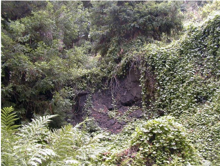
Figure 18 – Cape ivy has invaded the light gap created in the canopy by slope failure and tree-fall along Joshua Creek. November 2004.
