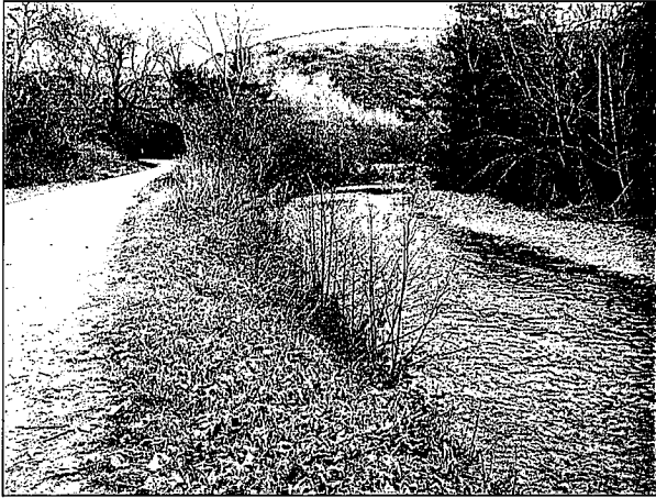
1997-98 Right bank failure at ranch road. (RM 1.29-1.32). Note alder and willow recruitment at toe. Road realignment and bio-engineered slope treatment proposed.
